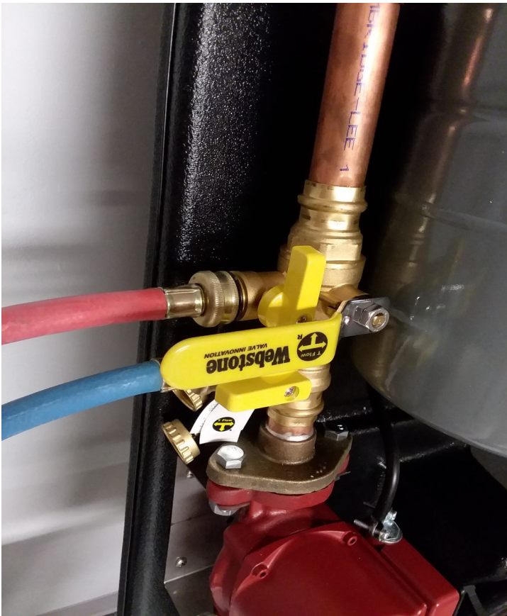
Valve Position to Pressurize the System
